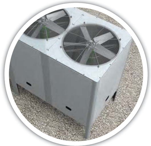
Remote condenser inlet air filters are easily accessible and washable.
